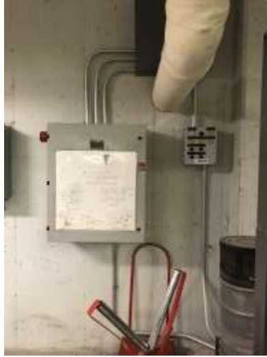
#1 OWS oil level alarm monitor panel on right
