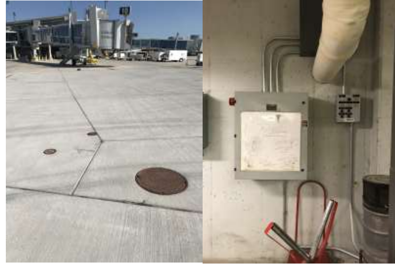
#4 Below grade Gate 10 OWS valves #5 Ancillary sump control panel/ OWS oil level alarm monitor panel
